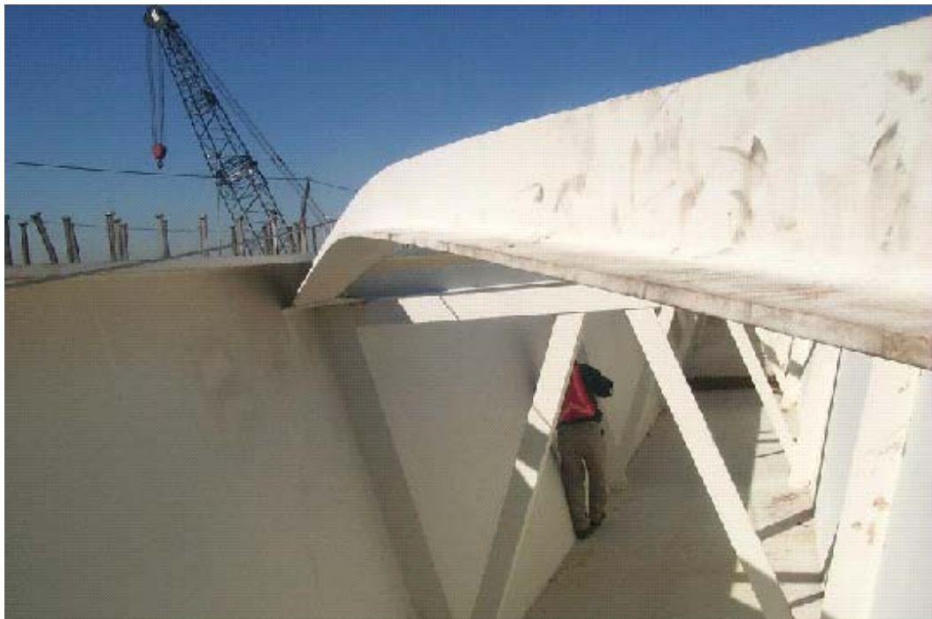
Figure 1.2 Local failure of bracing member during construction (Chen, 2002)
